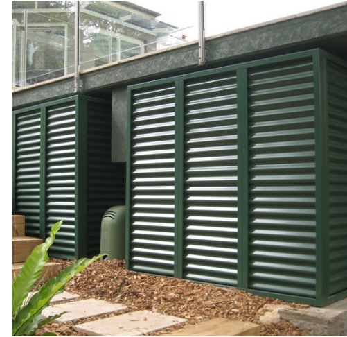
Figure 93: Concealed tanks integrated with the design.
